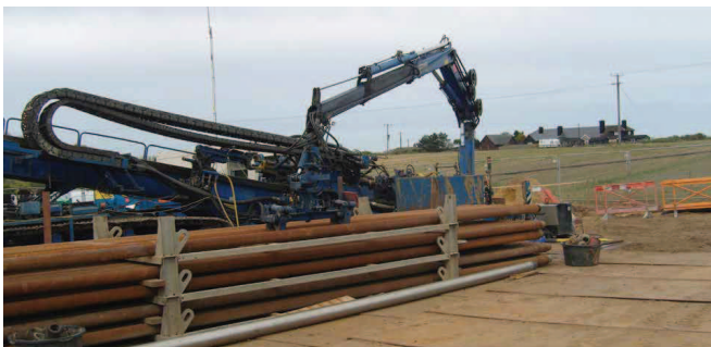
Horizontal directional drilling unit (HDD), showing the drill rig and drilling pipes.
